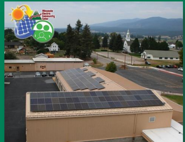
Photos: (Top) MEC Solar I; (Bottom) MEC Solar II
